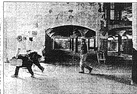
Construction workers pass Monday through an unfinished section on the ground floor of the former Tepper's department store on West Front Street in downtown Plainfield.
