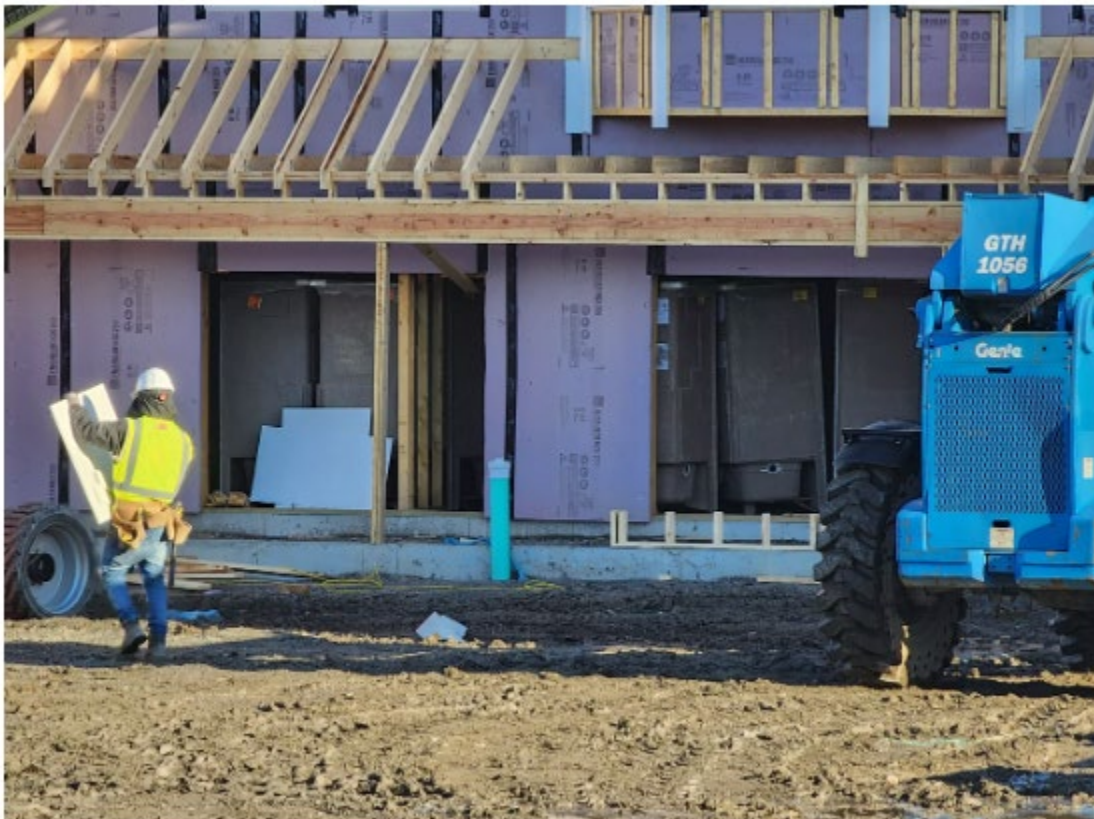
A worker at the Grand Avenue construction site on March 18, 2025. Photo: Bob Joseph/WNBF News
