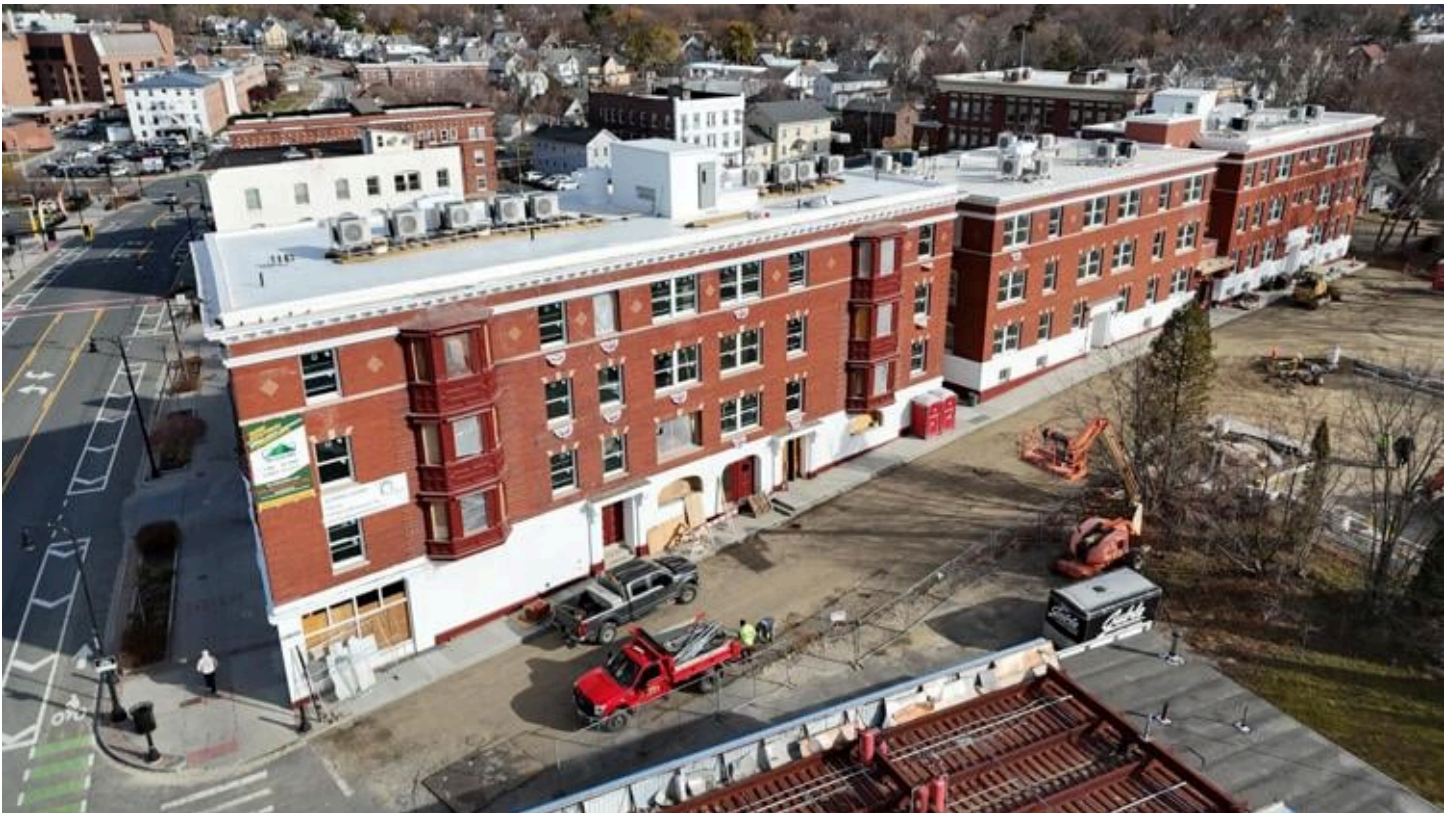
Terrace 592, formerly White Terrace, is in the final stages of construction, and will be ready for move-in by mid to late-April.
