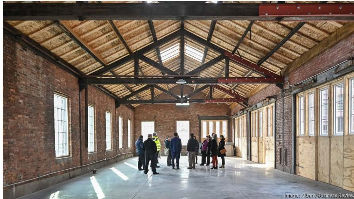
A former carriage house in the rear of the property that was in bad shape now has a new roof, skylights, doors, windows and concrete floor. The 2,100-square-foot building is available for commercial lease.
